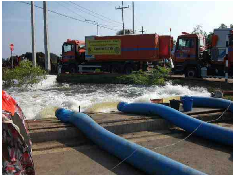
Discharging water (picture taken near Ayutthaya TC)
